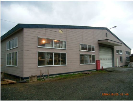
図 14 A'地点の工場の被害(A damaged wall of a factory building)
