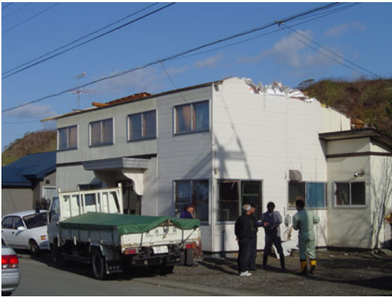
図 8 屋根小屋組の飛散(A damaged house whose roof frames was peeled off)
