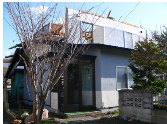
図7 2階部分の飛散した住宅(A damaged house whose 2nd floor was collapsed)
