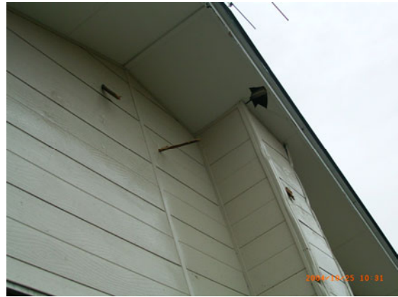
図 11 外壁への飛来物の衝突(Some windborne missiles and some traces on a wall of wooden house)
