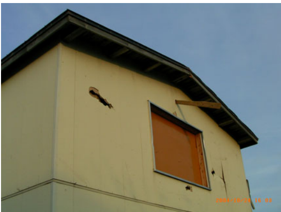
図 10 外壁への飛来物の衝突(A windborne missile and some traces on a wall of wooden house)
