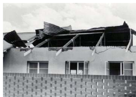
Figure 3b. Wind damage to a house
